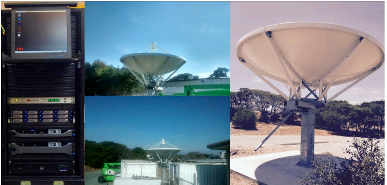
4.5m Capella-GR Ground Station and Indoor Equipment
